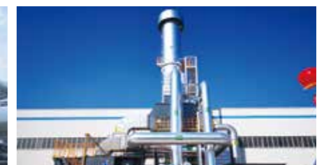
Waste gas treatment in engineering machinery coating Zeolite rotor + RTO
