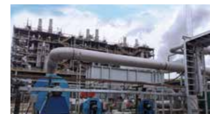
Treatment of organic waste gas in chemical plant 3-canister RTO
