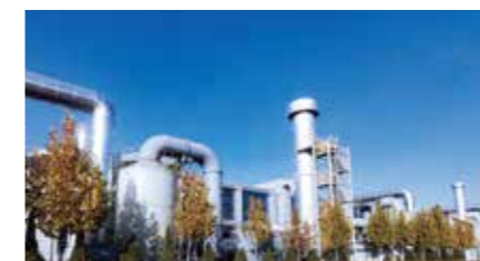
Treatment of acidic and alkaline waste gas in the tire industry Activated carbon + spray tower
