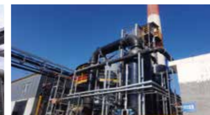
Treatment of organic waste gas in chemical plant Rotary RTO
