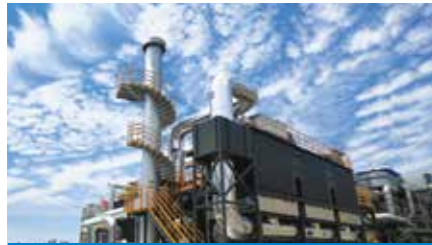
Treatment of organic waste gas from aluminum-plastic packaging 3-canister RTO
