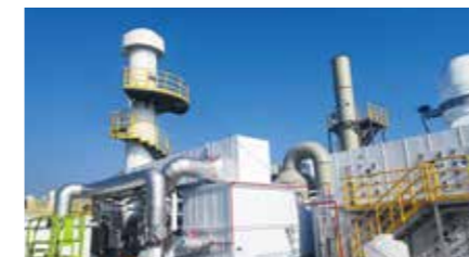
Treatment of VOCs waste gas in electronic industry Zeolite rotor + RTO
