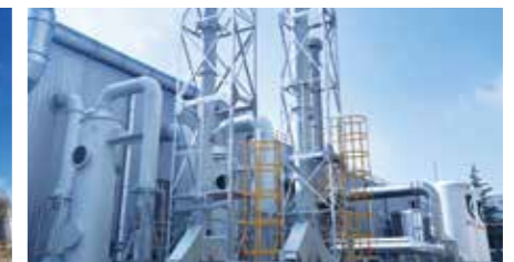
Treatment of acid and alkaline exhaust gases in the semiconductor industry Scrubber
