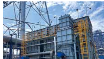
Fischer-Tropsch tail gas treatment 3-canister RTO
