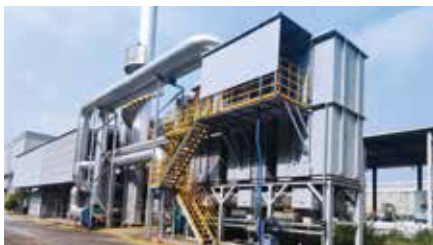
Treatment of organic waste gas in pharmaceutical production 3-canister RTO
