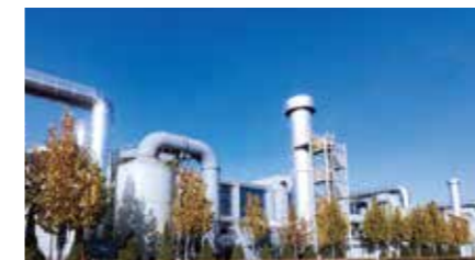
Treatment of acidic and alkaline waste gas in the tire industry Activated carbon + spray tower
