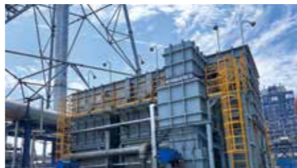
Fischer-Tropsch tail gas treatment 3-canister RTO
