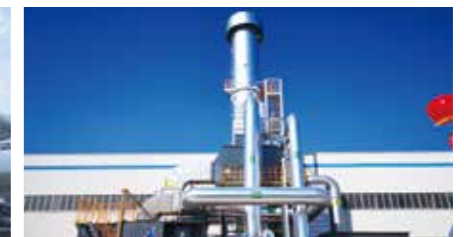
Waste gas treatment in engineering machinery coating Zeolite rotor + RTO
