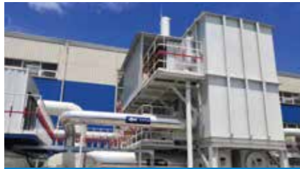
Waste gas treatment in ship manufacture plant coating 3-canister RTO
