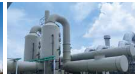
Treatment of acid and alkaline exhaust gases in the semiconductor industry Scrubber
