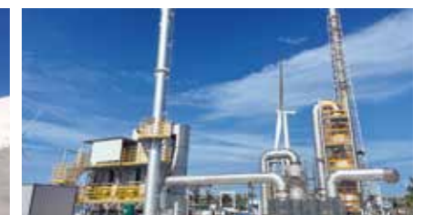
Treatment of organic waste gas from petroleum refining 3-canister RTO
