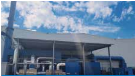
Waste gas treatment in ship manufacture plant coating Zeolite rotor + CO
