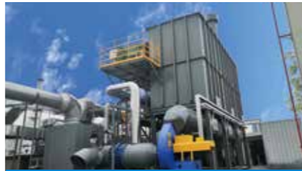
Waste gas treatment in 3C coating 3-canister RTO
