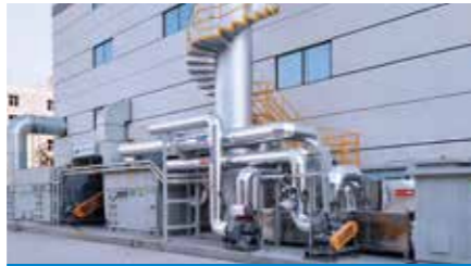
Treatment of organic waste gas in printing industry Zeolite rotor + CO
